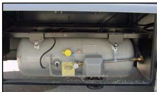
Figure 2-2. Liquid Propane Tank
