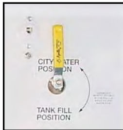
Figure 11-7. Water Fill Valve
