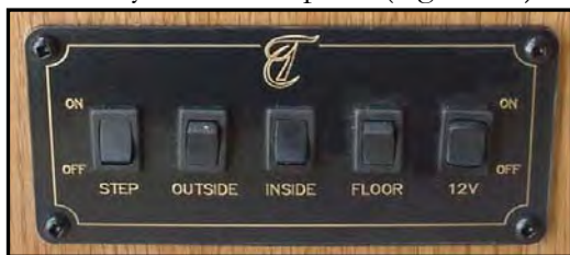
Figure 7-4. Battery Disconnect Panel
