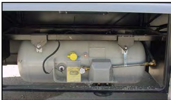
Figure 2-4. Liquid Propane Tank
