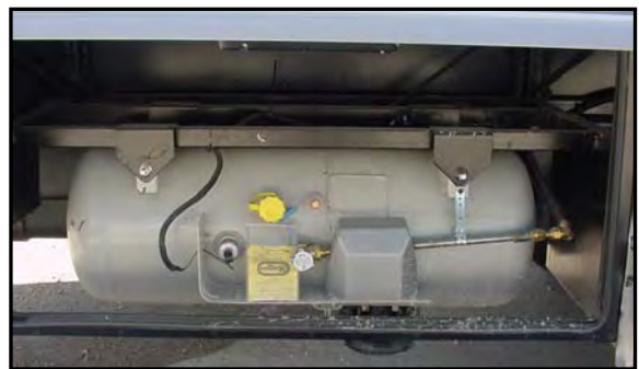
Figure 3-5. Liquid Propane Tank
