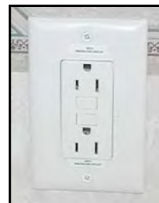
Figure 7-5. Typical AC Receptacle
