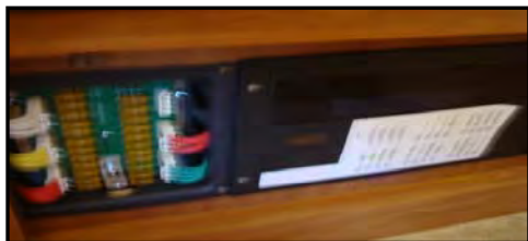
Figure 7-1. Circuit Breaker Box
