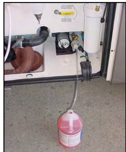
Figure 13-17. Wintering Process for the Motor Home
