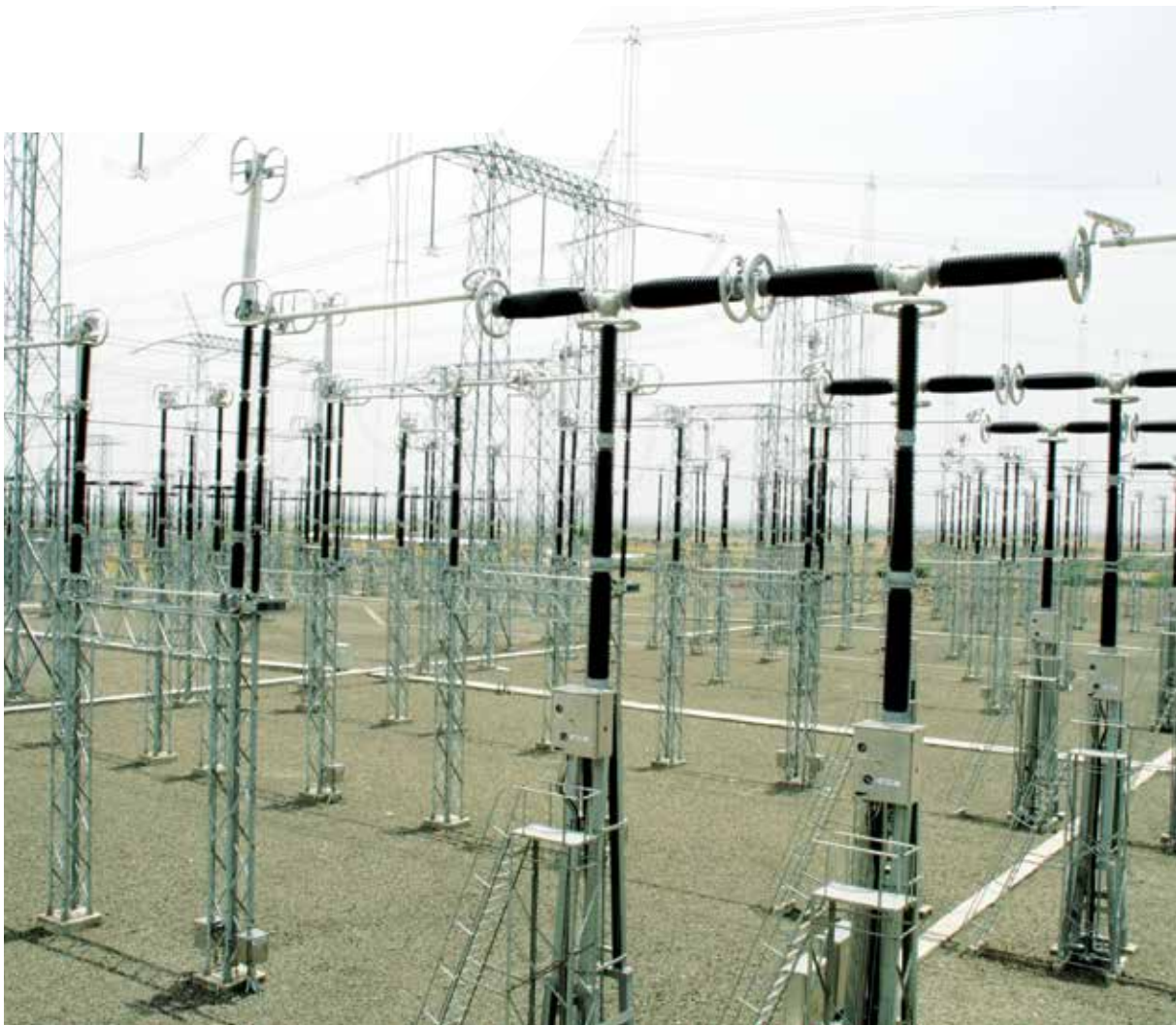
765/400kV Air Insulated substation at Dhule, Maharashtra for Sterlite Transmission Limited
