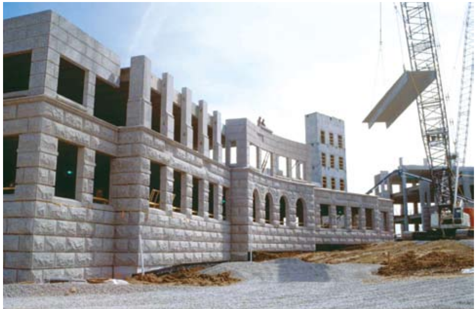
The all-precast concrete structural system includes double tees, inverted tee beams, shear walls, and loadbearing precast walls. The system is a common approach to design in the Rocky Mountain region.
