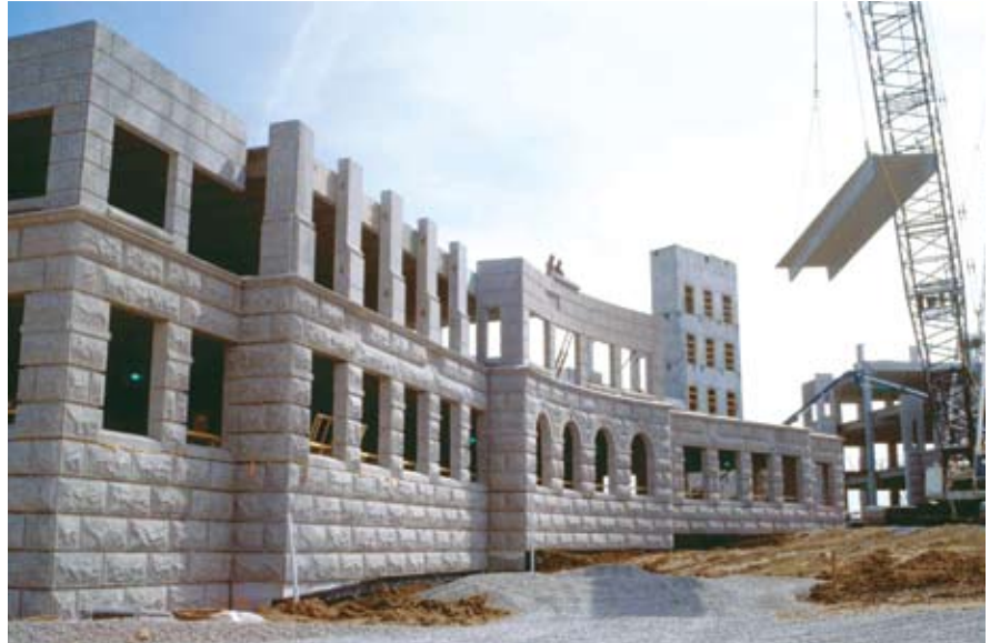
Starz Encore headquarters all-precast structural system includes shear walls, loadbearing precast walls, double tees, and inverted tee beams. The system is a common approach to design in the Rocky Mountain region.
