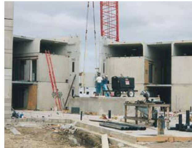
Two converging wings of Special Housing under construction expose the precast components of the building; stacked modular cells, hollow-core slab corridors, plenums, and insulated wall panels.
