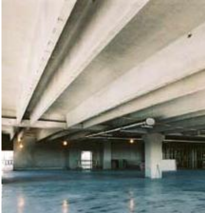
The Enterprise IV project features double tees as flooring, which create large, open floor plans that add flexibility for tenants.
