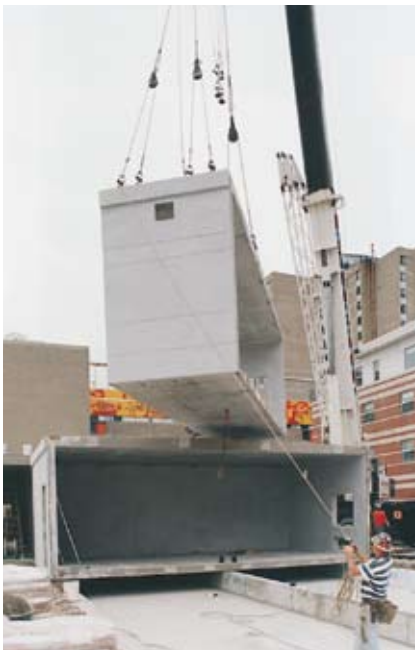
A crane hoists one of the 30-ft modules into place on the concrete foundation. The modules were delivered at night under a police escort because of daytime congestion in the area.
