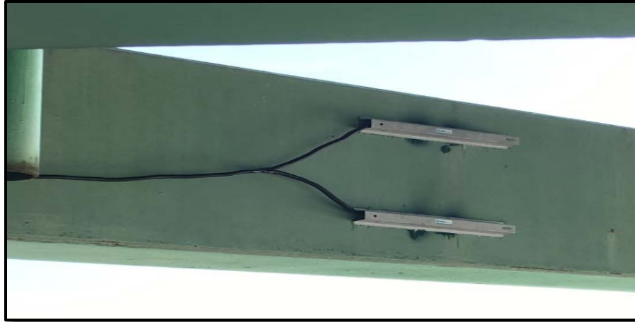
Figure 6.7 - Steel Gage Covers
