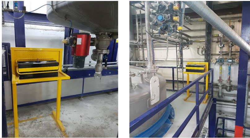
Fig. 9. Tool box fixed nearby work centers.
