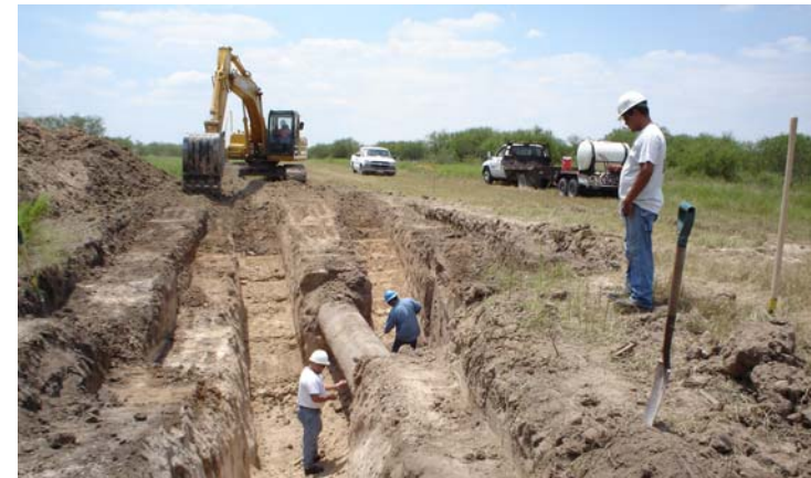
Confirming and mitigating external corrosion detected by ILI
