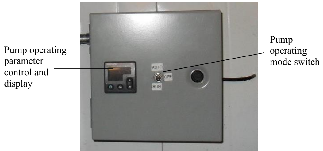
Figure A.26– Temperature controller for freezer chamber pump #2
