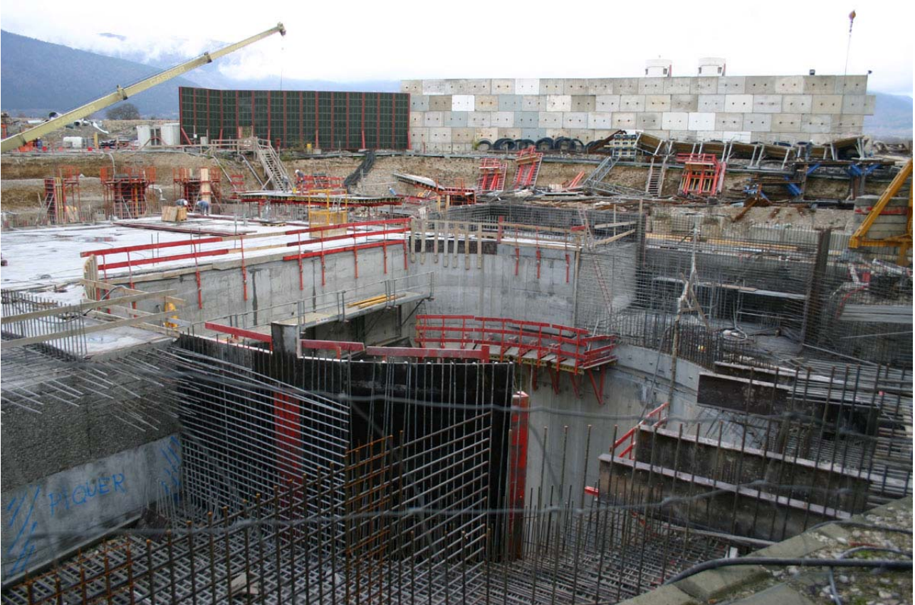
The PX56 access shaft. The concrete surface is being constructed, in preparation for lowering pieces of CMS.
