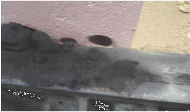
Fig.6: Improperly Sealed Runner Bar End
