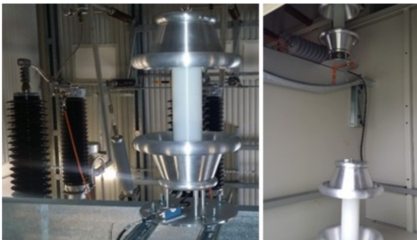
Figure 1 Voltage sensors in substation and in A11
