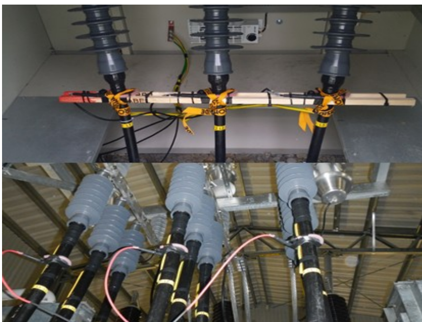
Figure 2 Current sensors in A11 and in substation
