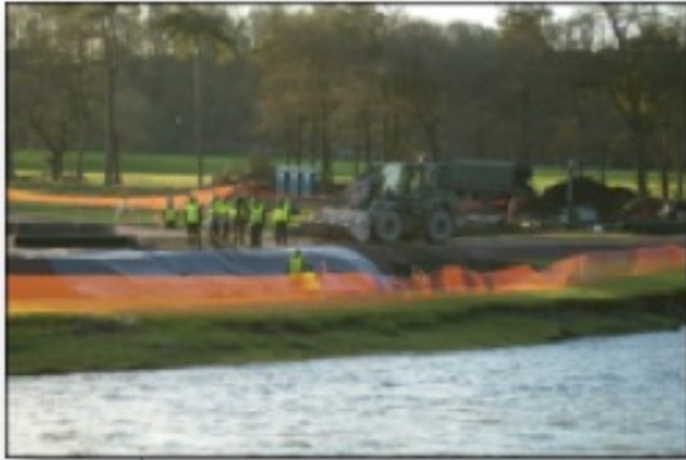
Cumbria Floods – November 2009 Workington Bridge, Cockermouth
