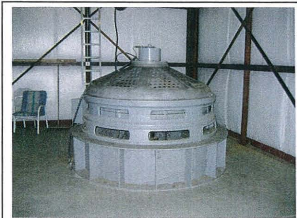
Hydropower turbine/generator at Pristine Springs
