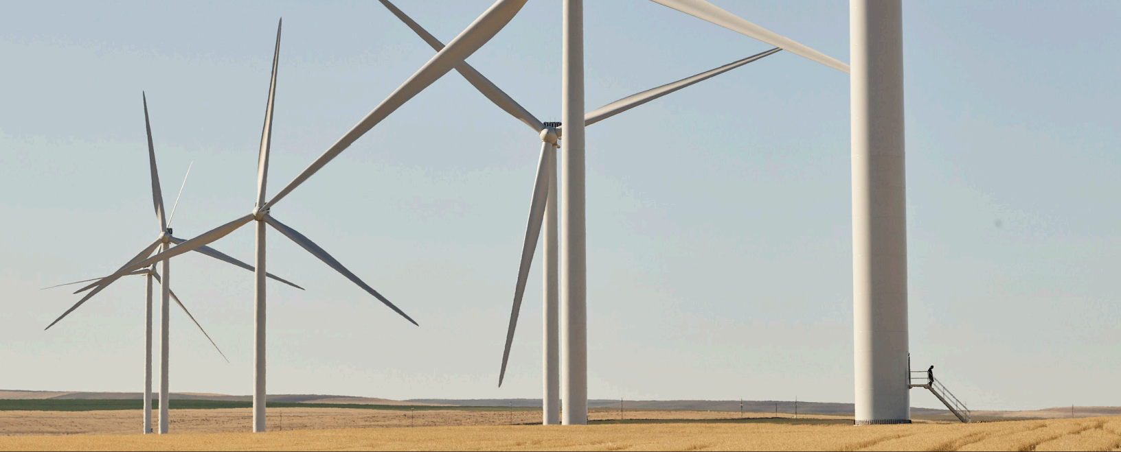
The Montague Wind Farm supports our Prineville data center producing over 560 million kWh of renewable energy a year.
