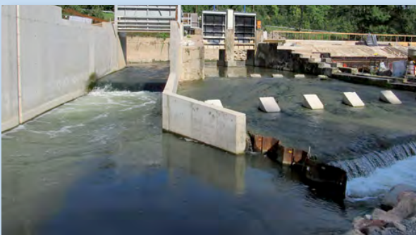
A field test began in the summer of 2013. A conventional small power station was set up in a branch of the river Tauber close to the Bronnbach Branch Office of the Fraunhofer ISC.
