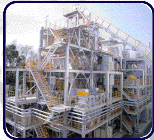
A pilot plant for gasifying melting incineration system in Sodegaura, Chiba Prefecture, has been in operation since April 1998.
