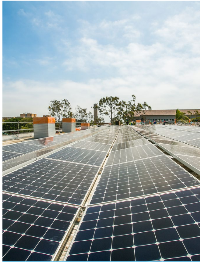
Solar panels at UC Santa Barbara
