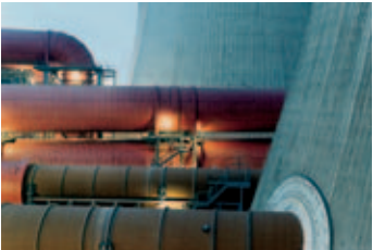
Purified gas lines leading to cooling towers
