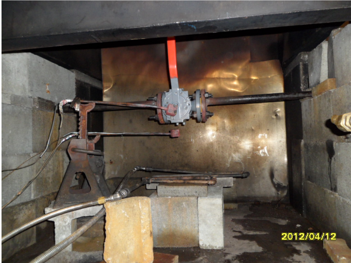
Test Valve Prior to Burn
