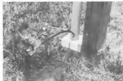
Fig 3—The base of the driven element. The wire projecting from the ground rod and almost touching the base of the antenna element is the horn (air) gap for lightning protection.
