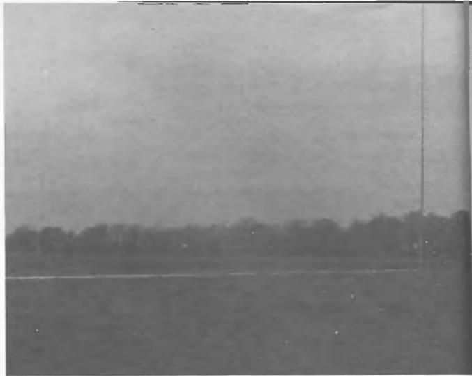
Fig 9—The array installation for 80- and 40-meter operation using Butternut HF2V verticals.
