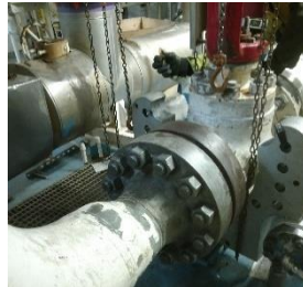
Recomissioned system post AOGV operation
