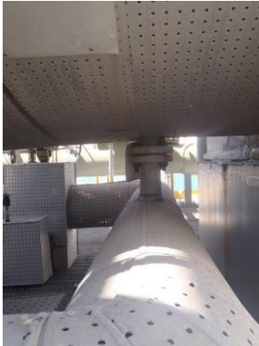
Slug catcher isolation Cryogenic -163 deg C
