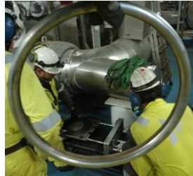
Gasket removed from live 150 HC Gas system
