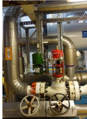
Control valve isolation Gas export
