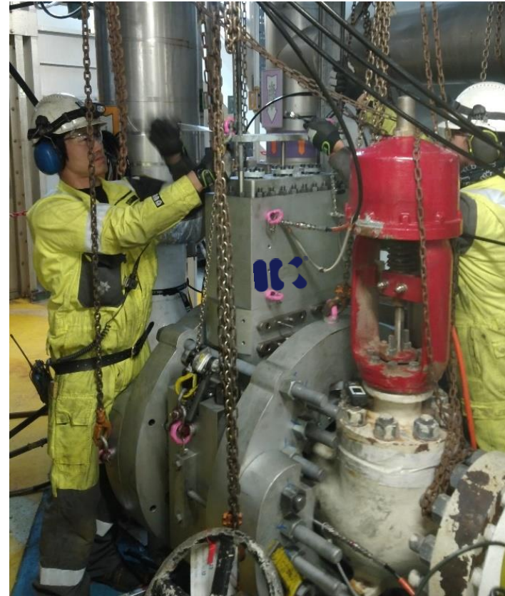
AOGV operation ongoing
