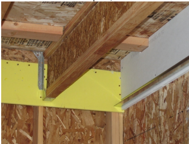
Figure 5.3.2 – Use of joist hanger to reduce amount of cross grain wood shrinkage.
