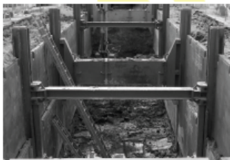
Unstable Soil Conditions
