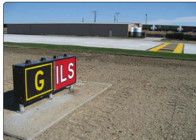
Figure 1-36. Instrument landing system (ILS) holding position sign and marking on Taxiway Golf.
