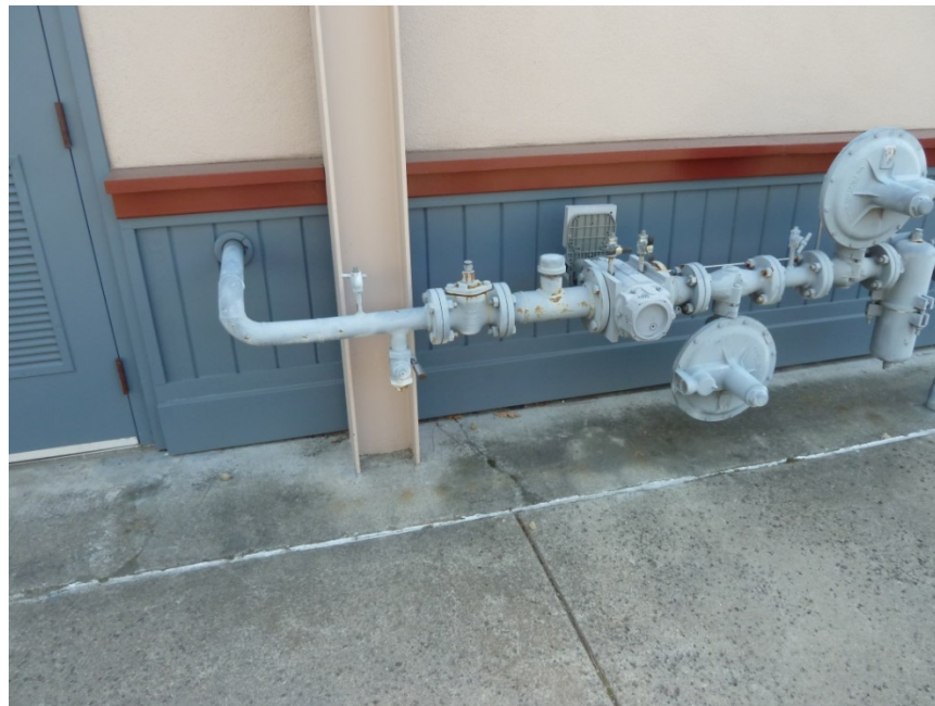
Existing Gas Meter
