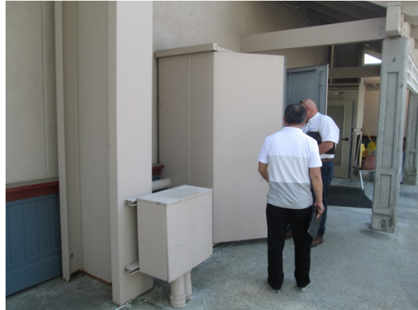
Existing Main Switchboard closet and distribution board closets.
