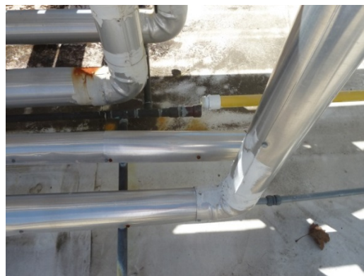
Condensate drain disconnected
