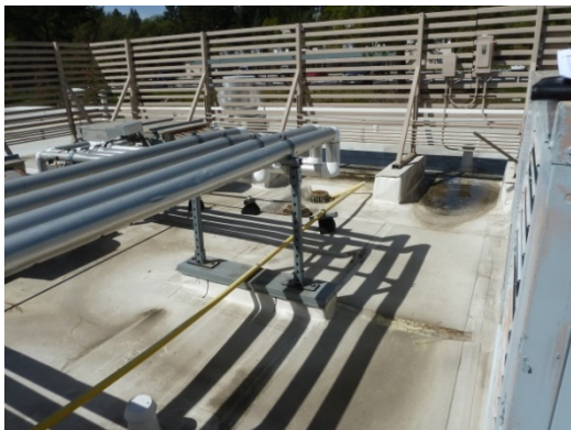
Corrosion at drain domes
