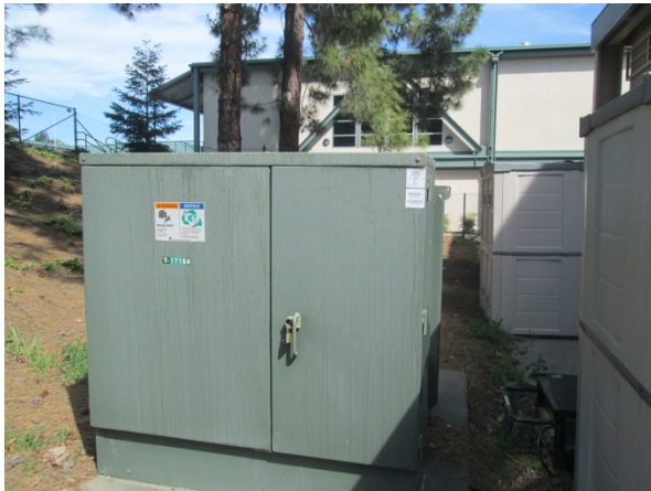
Existing PG&E transformer
