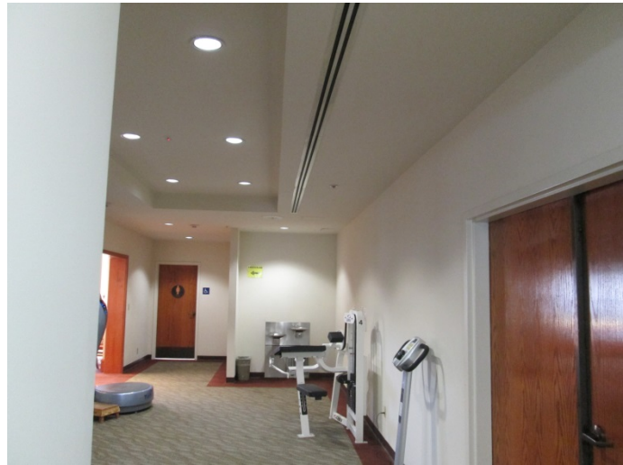
Existing lighting showing scalloping on walls
