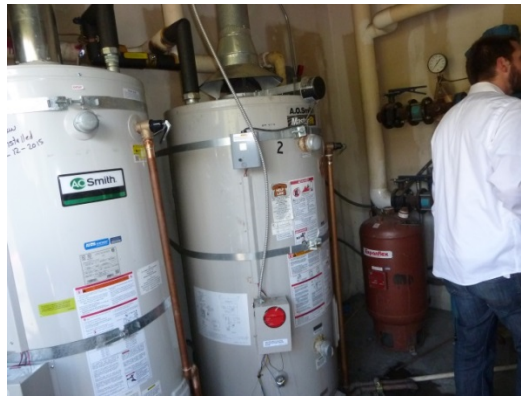
Existing Domestic Hot Water Heaters
