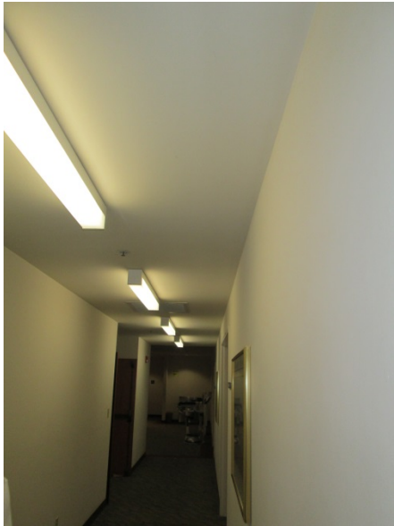
Existing corridor lighting
