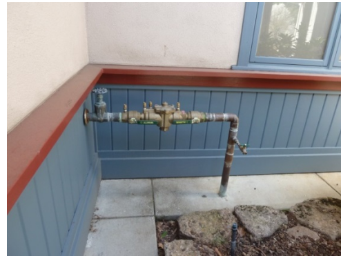
Irrigation Backflow Preventer
