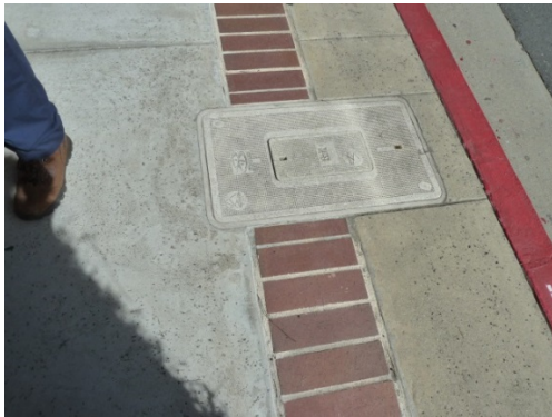
Domestic Water Meter in Vault
