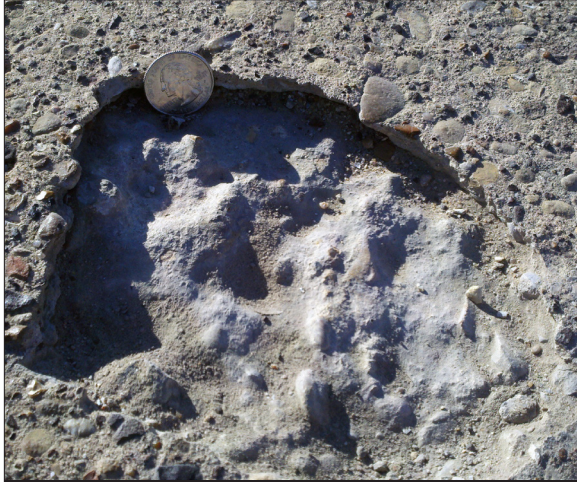
Pit in concrete
