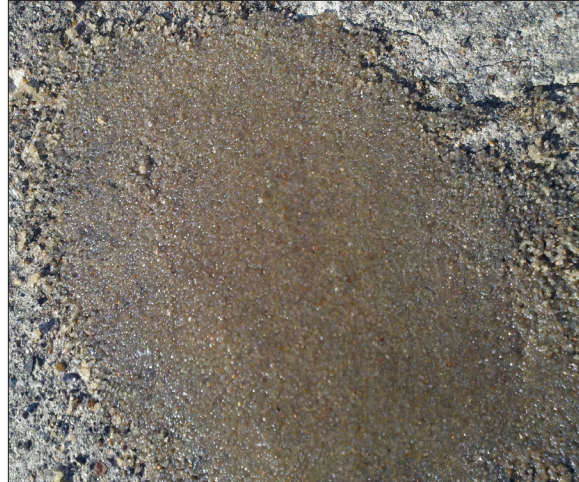
Pit patched with epoxy and sand
