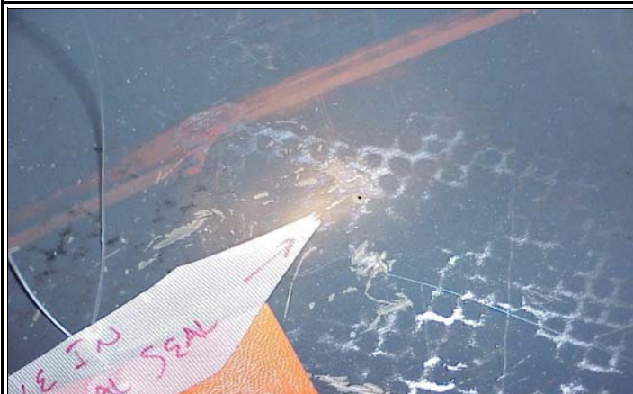
Figure 2. Close-up of hole in the STS-92 vertical stabilizer caused by collision with a stainless steel debris particle.
