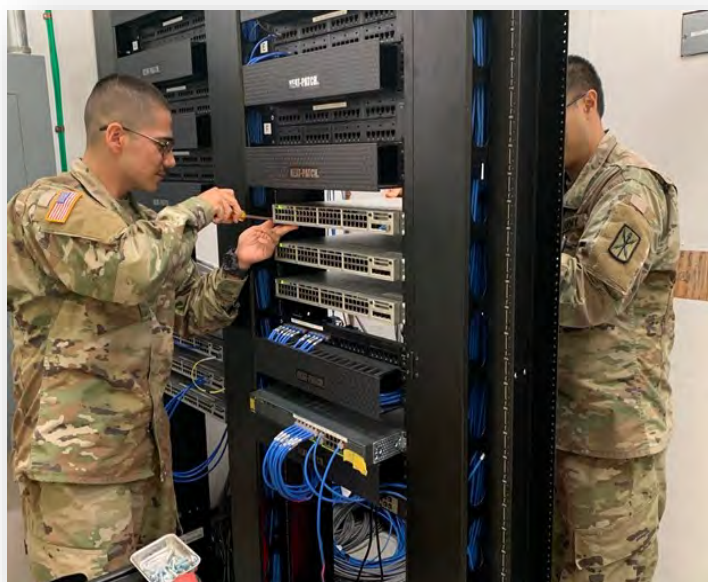
USANEC-O Soldiers from the Network Support Branch, Pfc. Carlos Garcia (left) and Spc. Victor Nguyen, learn how to install and configure switches during the telecommunications installation of the new Network Enterprise Center. (U.S. Army photo by Staff Sgt. Jennifer Monge/Released)
