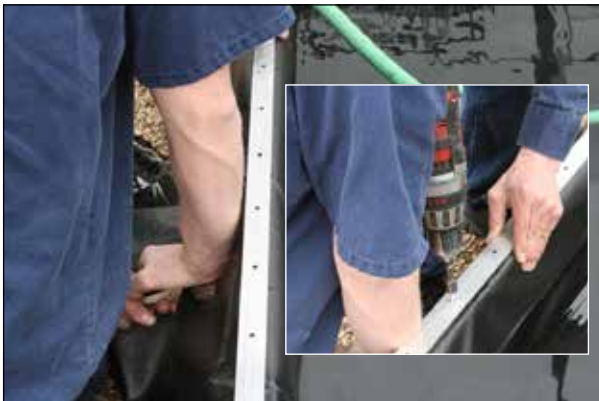
4. Apply slight downward force to stretch liner material and secure strap with Tek screws.
