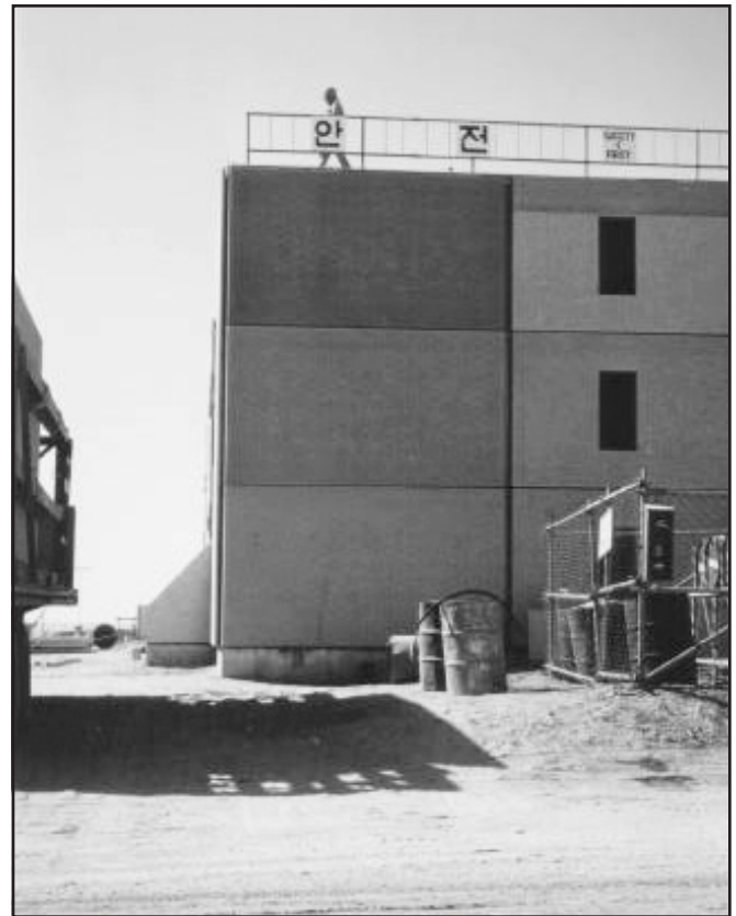
Figure 4-1. Color variations in precast panels due to use of different cements
