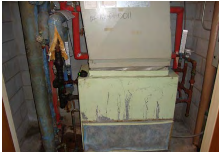
Figure 4.2: Belk Hall – Air Handler for Suites, in Mechanical Closets
