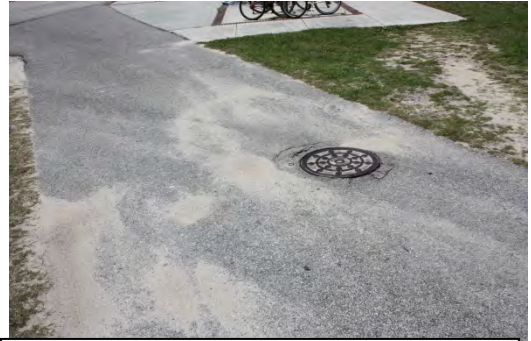
Cracking around Manhole
