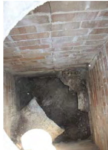
Cracking inside stormwater manhole
