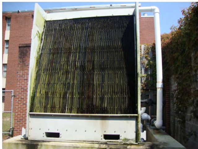
Figure 4.1: Cooling Tower with Algae Formation.
