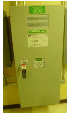
Figure 5.8 Graham-Hewlett Transfer Switch
