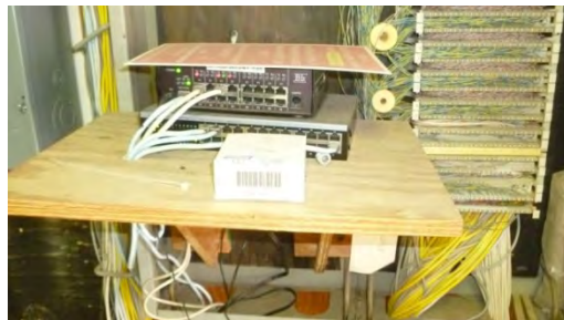
Figure 5.10 Telephone and Data Equipment in Mechanical Space
