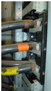
Figure 5.6 Typical Feeder Termination
