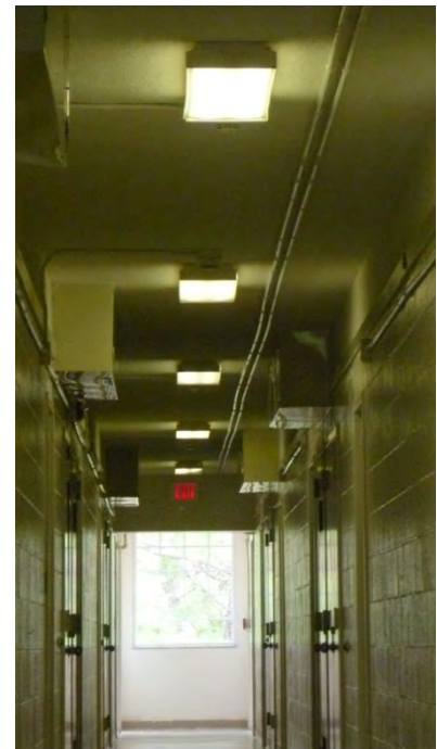
Figure 5.3 Hewlett Corridor Emergency Lighting
