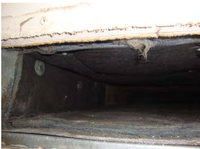
Figure 4.4: Supply duct with liner, Can be Cleaned and Encapsulated
