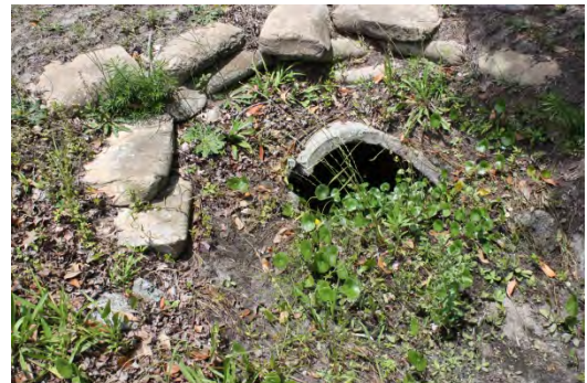
Discharge from parking area to ditch
