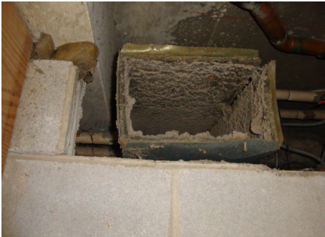
Figure 4.3: Return duct with liner, recommended to be replaced
