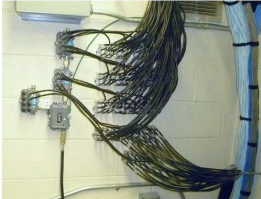
Figure 5.14 Typical CaTV Splice
