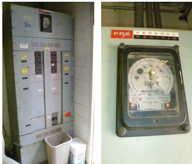
Figure 5.5 Graham Hall Main Service Panel and Meter
