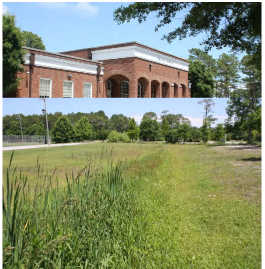
Overgrowth of vegetation in drainage ditch
