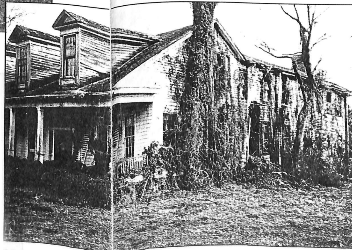
Before the Dents could begin restoring the 147-year-old house, they had to cut away trees, bushes and vines that had grown up around the place. A wing at the back of the house (to the far right in this photo) had to be razed.
