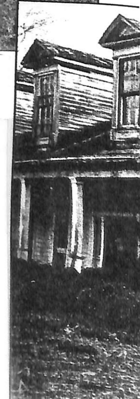
Before the Dents could restore the house, vines that had grown up had to be razed.
