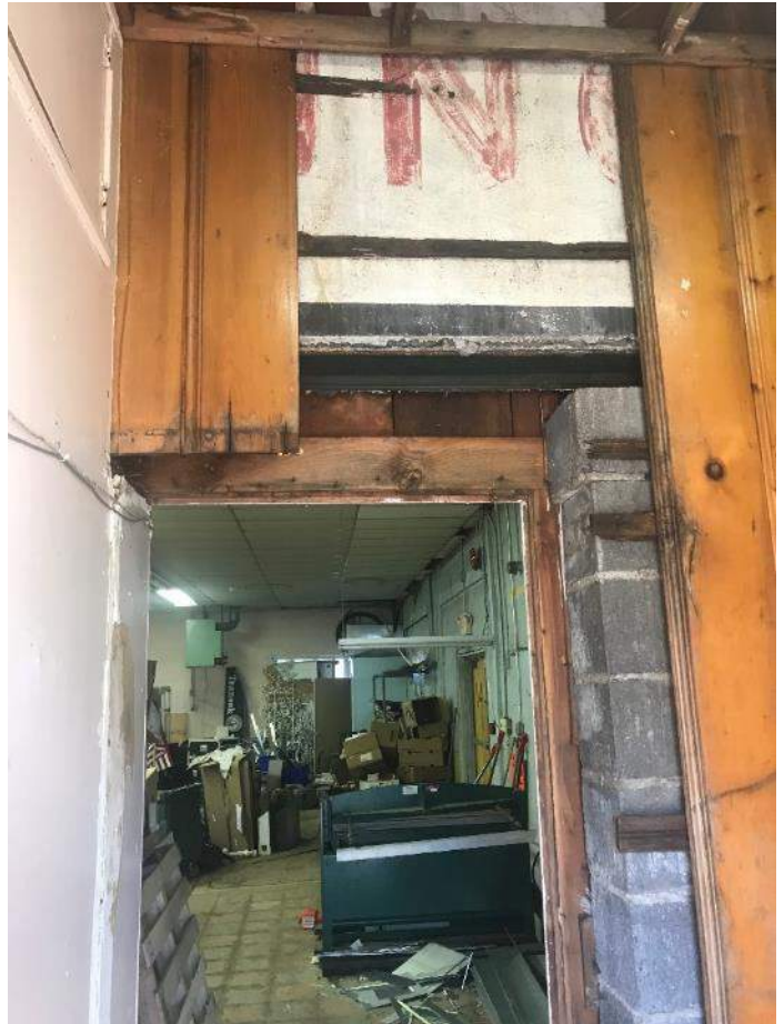
Interior - Substandard structural conditions
