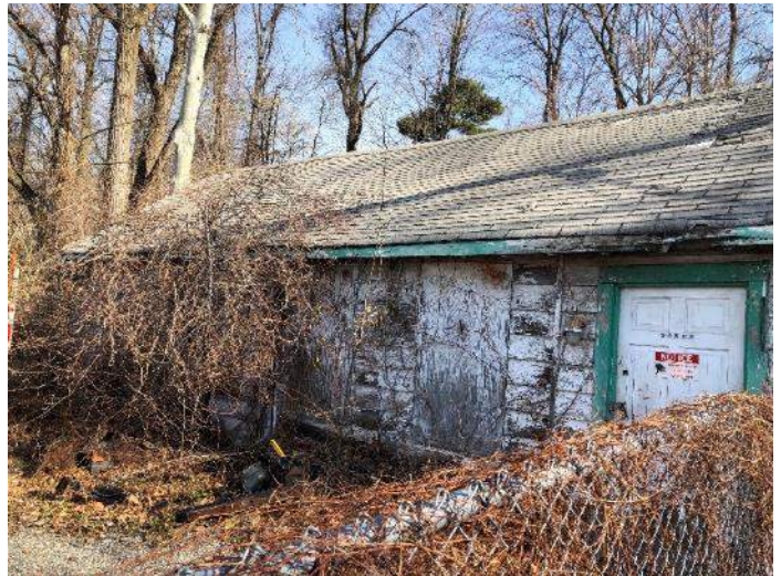
Wood frame structure in poor condition
