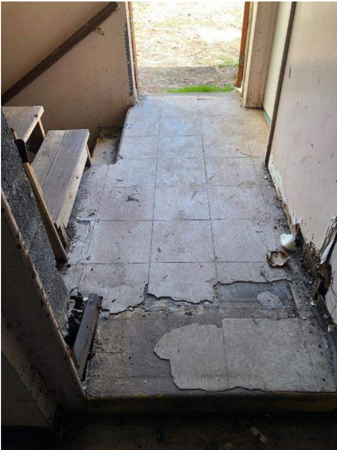
Interior - Cracked/dilapidated flooring
