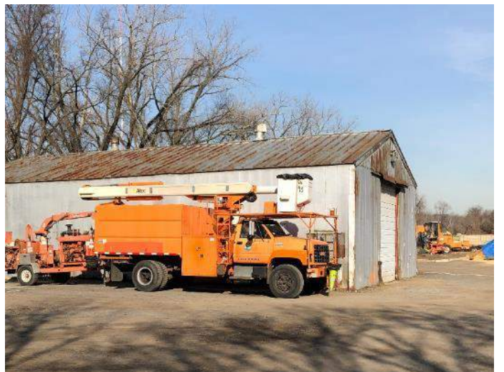
Exterior - Rusted garage storage structure
