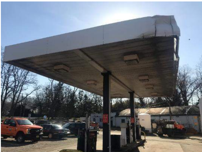
Fueling canopy and pumps
