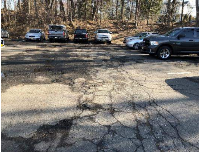
Cracked pavement and pooling in parking area
