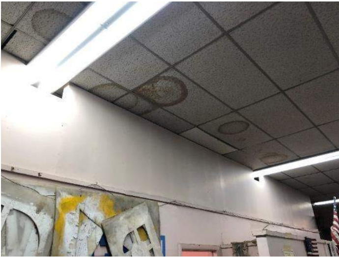
Interior - Water damage present on ceiling
