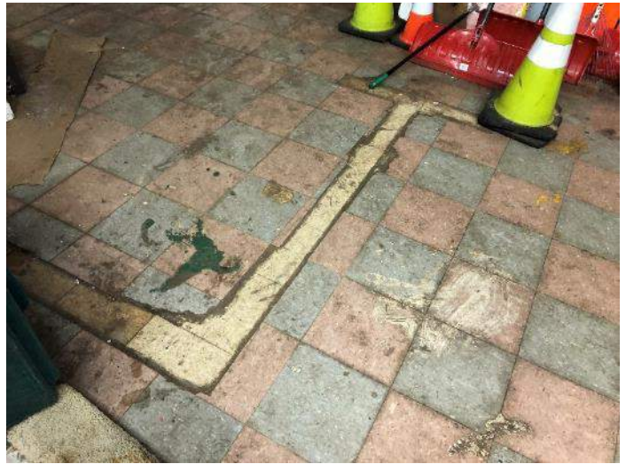
Interior: Cracked/dilapidated flooring
