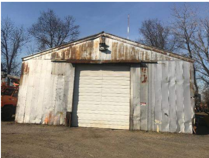
Exterior - Rusted garage storage structure
