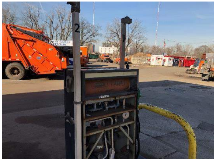
Detail of fueling pump
