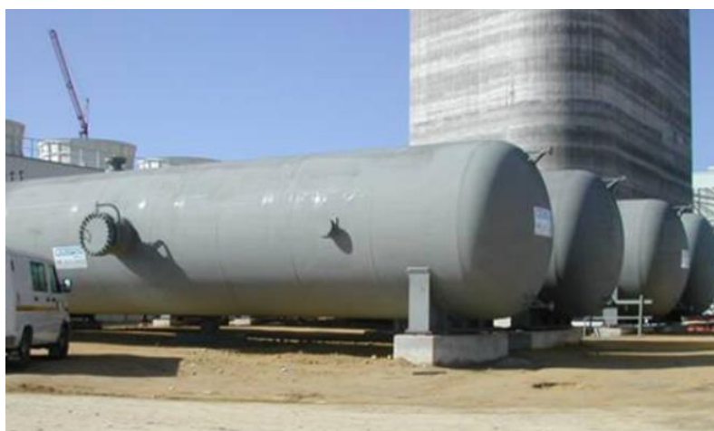
Figure 132: Steam accumulators at the PS10 Abengoa solar tower plant in Seville, Spain. (Reproduced from pole-derbi.com).
