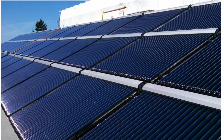
Figure 109: Evacuated tube collector array. (Reproduced from stage3renewables.com ).
