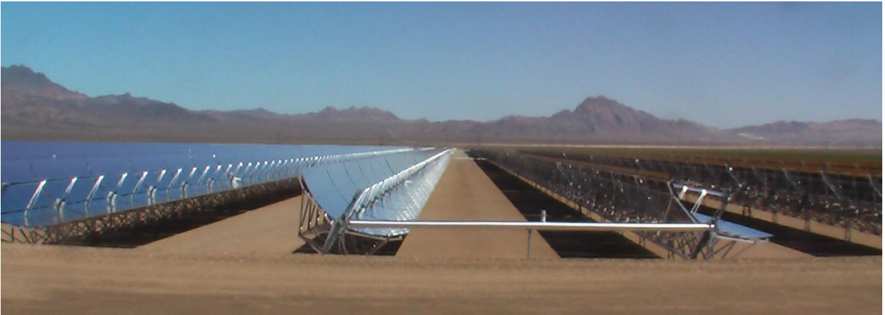
Figure 112: Parabolic trough field in a large CSP plant (image K. Lovegrove).
