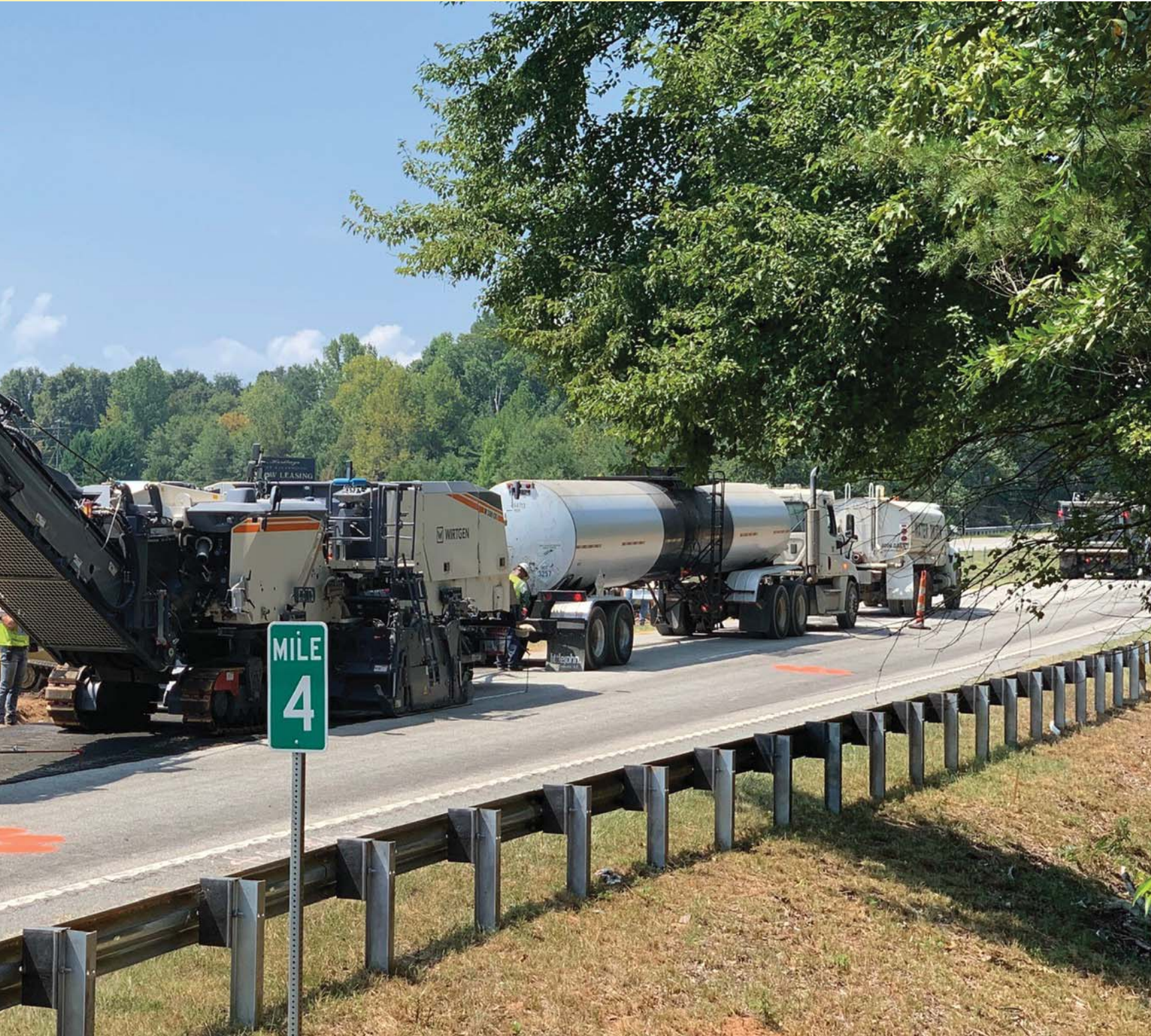
In a remarkable feat of speed, King Asphalt was able to complete the CIR portion of the U.S. 123 project—all 228,000 sq yd of it—in only 32 working days, which accounted for both weather-related and Clemson University athletics-related non-work days.
