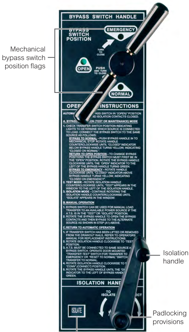
Mechanical isolation handle position window (connected/test/isolate)
