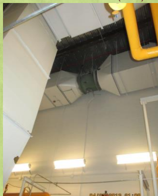
Return fan located 30 ft (9 m) off floor
