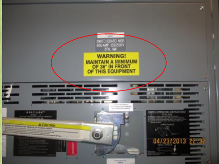
800 AMP service panel
