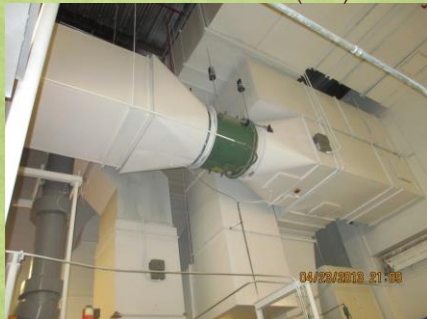
Return fan located 20 ft (6 m) off floor
