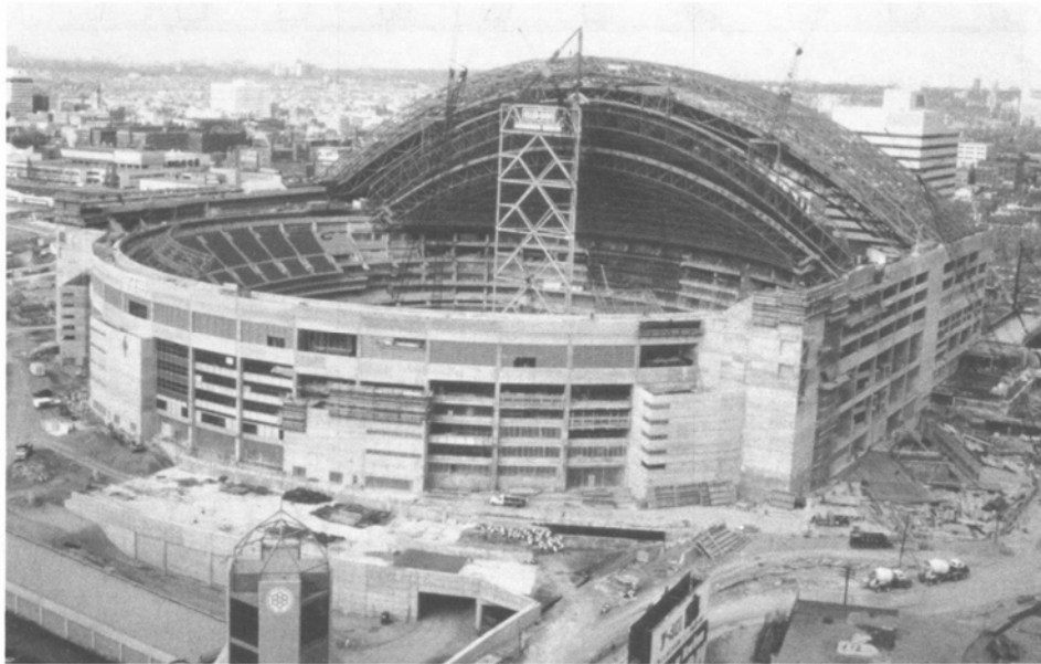
Fig. 27 SkyDome construction nearing completion. Courtesy of Jane Welowszky, SkyDome Stadium Corporation of Ontario
