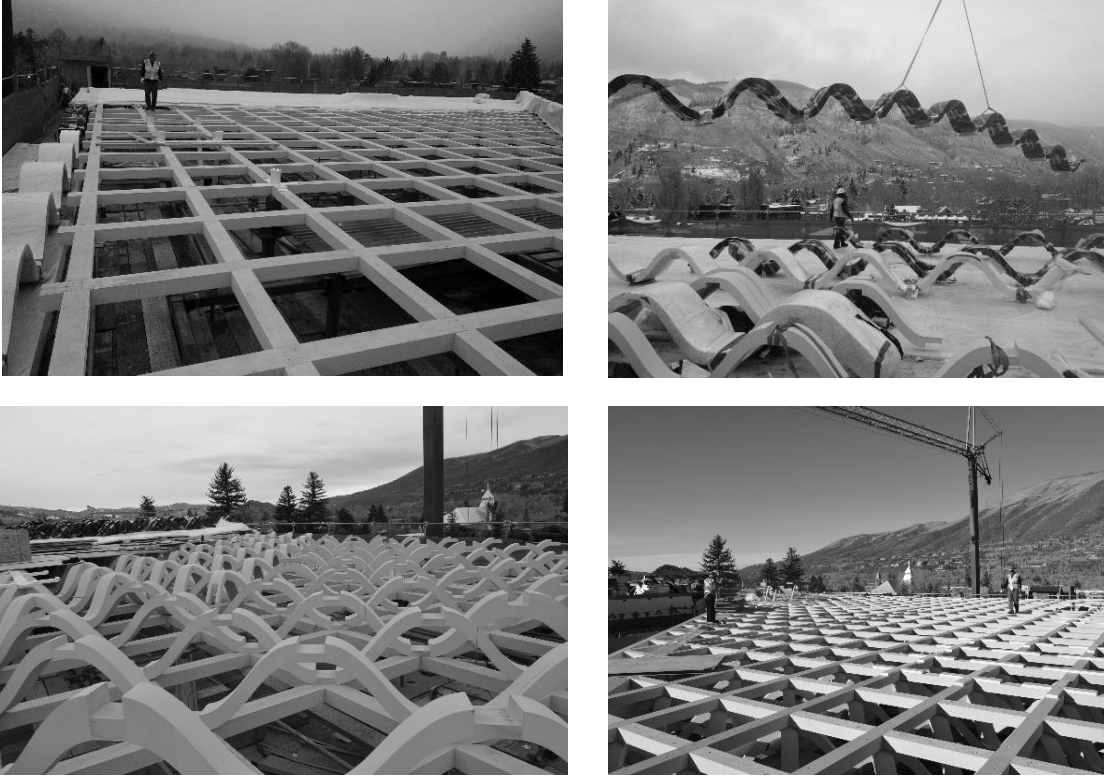
Figure 14: Construction of the truss, showing the bottom chord layer, the web layer, and the top chord layer at each phase of construction.
