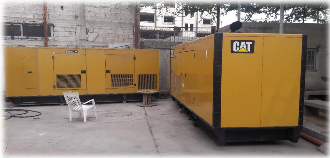
Figure( 3-5): Generators in Pumping Station.
