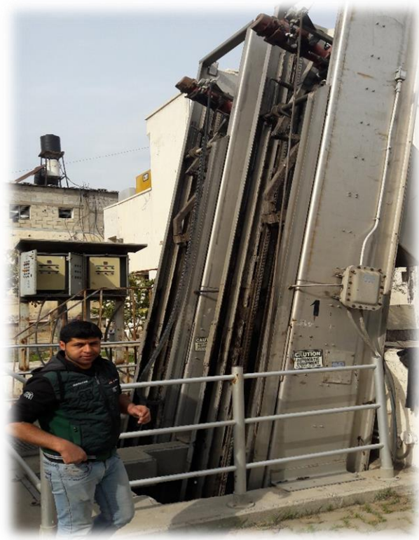
Figure( 3-4): Bar Screen in Pumping Station
