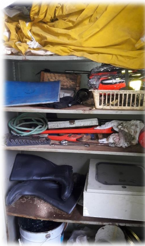
Figure( 3-7): PPE in Pumping Station.
