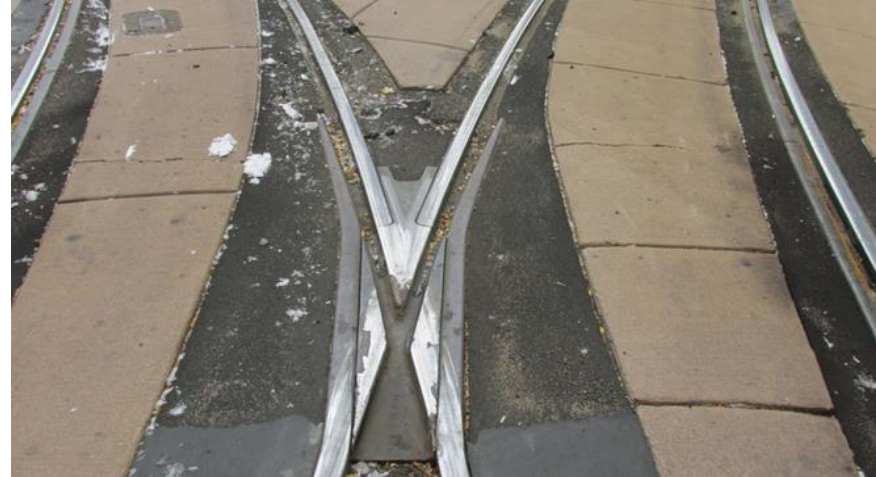
Not in a State of Good Repair
