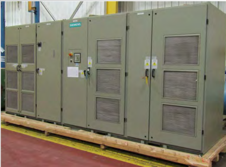
SIEMENS 1400KW HARMONY DRIVE VFD
