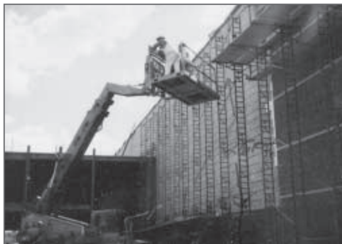
Fall Risk —This rough terrain forklift truck scaffold is missing a guardrail and there is no fall arrest system.
