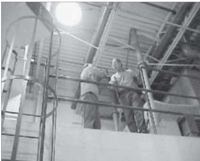
CET Consultant Lee Jay Kueppers is doing a follow-up to a hazard survey at L & L Products South Plant, to assure proper barriers are in place.
