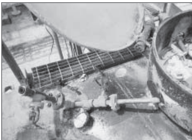
On top of the methyl mercaptan tank car, the broken unloading pipe is shown in the position it was found after the accident.
