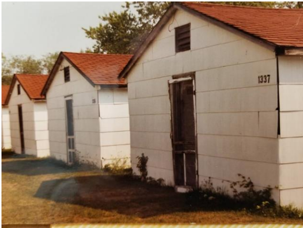
The old Huts. From what I have been told the roofs leaked, rodents living in them and very crude.
