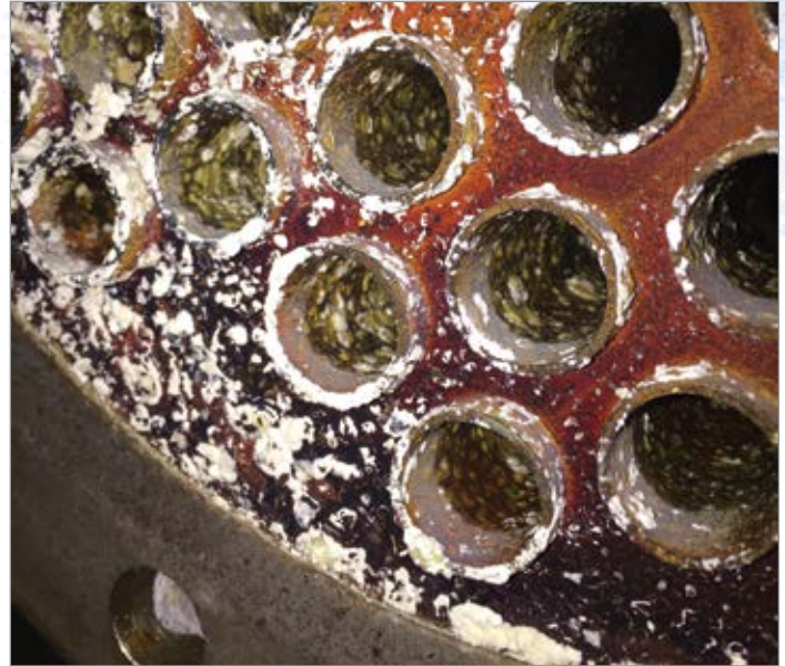
Figure 1: Severe fouling of water cooled condenser tubes.
