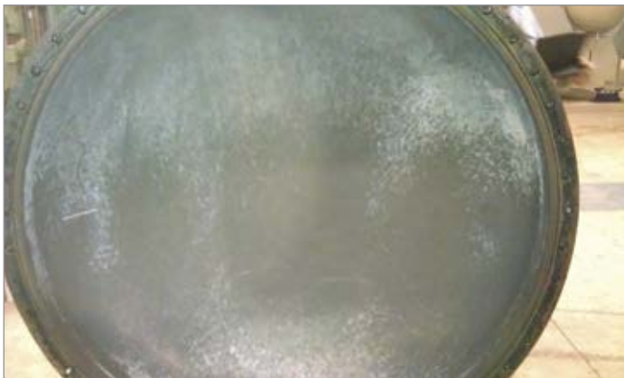
Figure 4: A view of the condenser shell end
