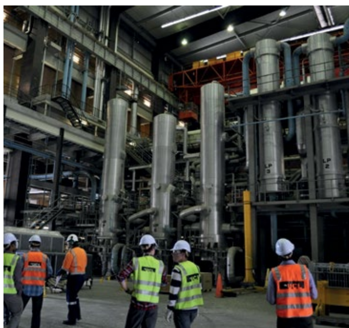
Figure 7: Coal and gas power stations, such as South Australia's Torrens Island gas power station (pictured), are responsible for most of Australia's electricity sector emissions.
