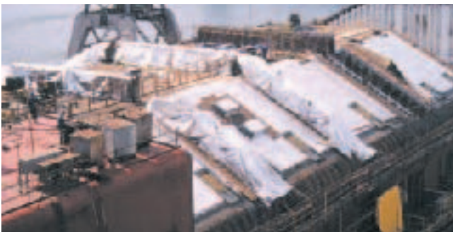
Figure 4. LPG carrier about half way through the production process. On the left-hand side, the top side of the carrier has been attached. On the right, the tanks (covered with insulation material) are still visible.
