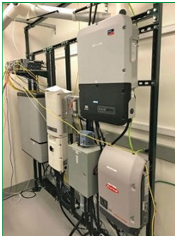
figure 9. The inverters under test in the ARPA-E NODES experiment. (Source: NREL; used with permission.)
