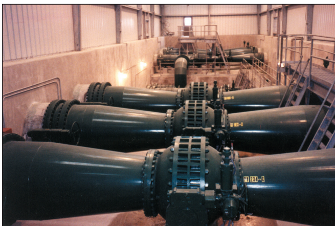
Ball valve in distribution pump station.
