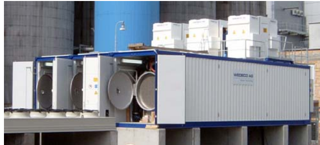
Figure 8 - Z-Compact-Systems delivering ozone to a bleaching fiberline
