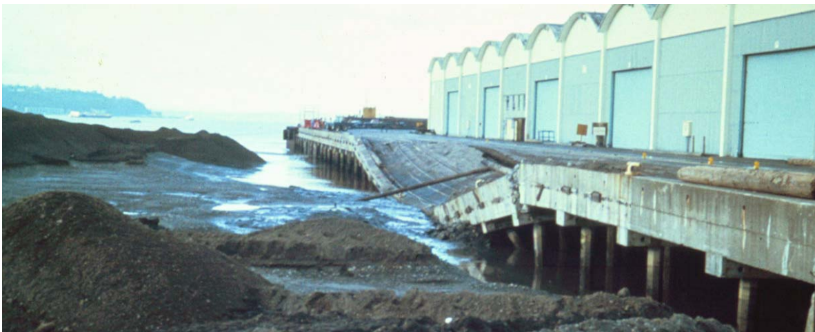
Fig. 7.15 View of the consequence of a hydraulic fill of fine silt flowing against 24-inch piles
