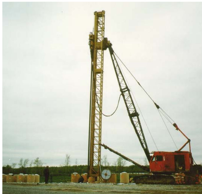
Fig. 4.5 Installation of wick drains type Alidrain (courtesy of J.C. Brodeur, Burcan Industries Ltd.)
